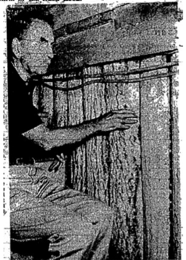
Mr. Healy shows how logs split in half were used in building some of the old house. The flat side was used for the kitchen and then lathing was nailed on for plastering. In the cellar, the round side of the logs was left uncovered.
